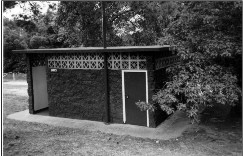
Buildings – some not very glamorous, but lots of them and important to the community – long life but high maintenance
