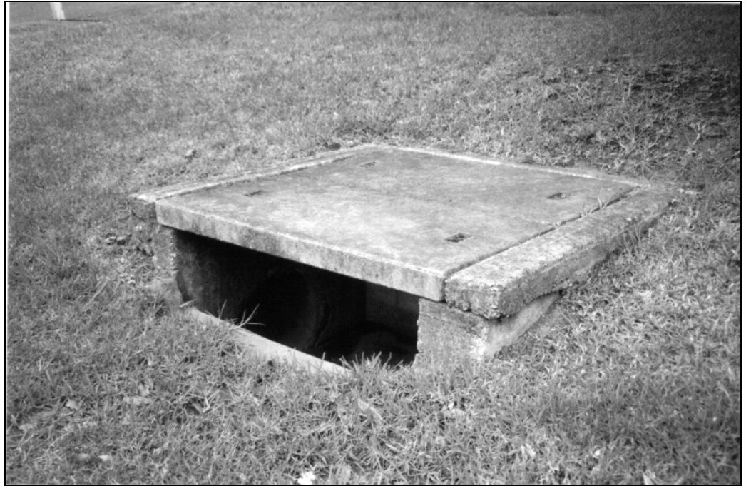
Typical drainage assets – much less volatile than roads, but harder to measure
